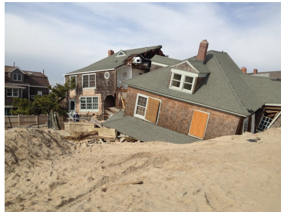
(b) Wave damage: houses break in the middle
