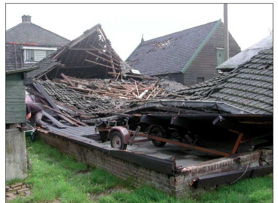
Figure 5. Damage of a (old) barn due to the tornado in Muiden on 23 August 2004 (photo by R. Sluijter).
